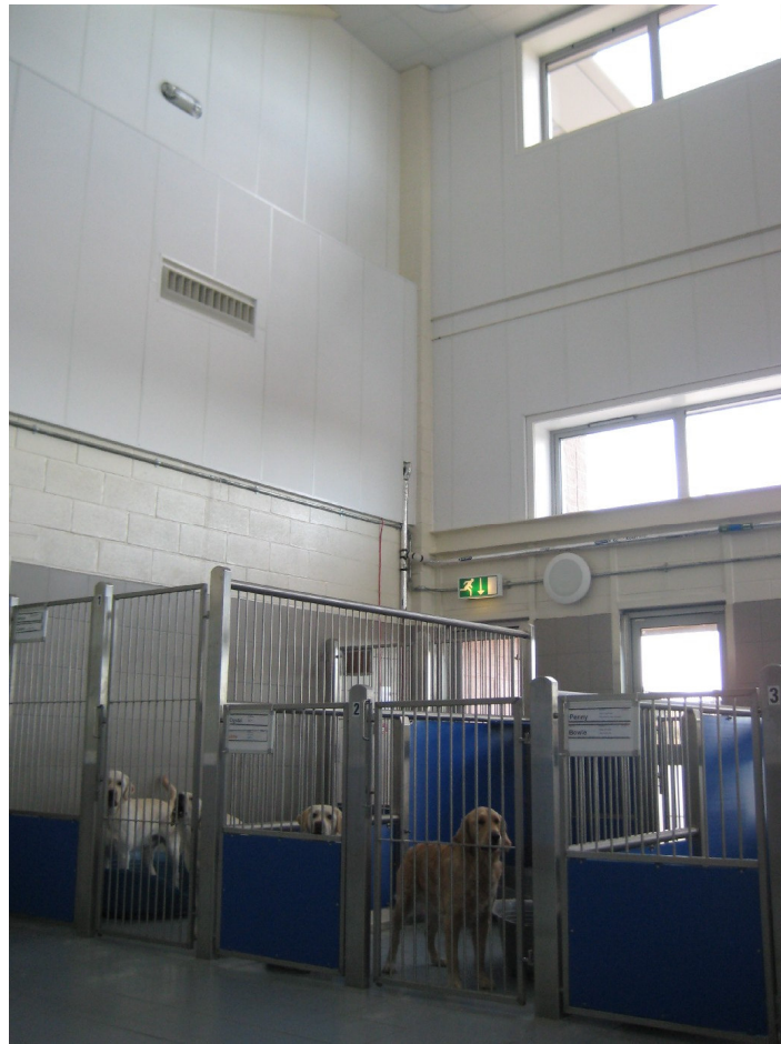
Figure 6: Glen Esk kennel block with additional absorption installed
